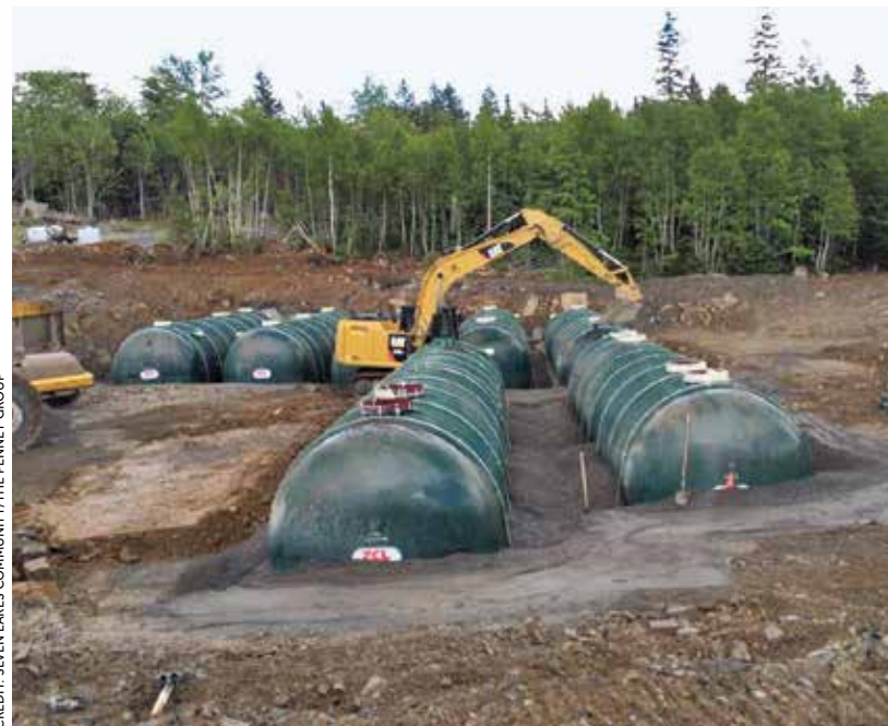
Repeat performance. Massive storage tanks store wastewater until it can be biologically broken down and used to recharge groundwater.
