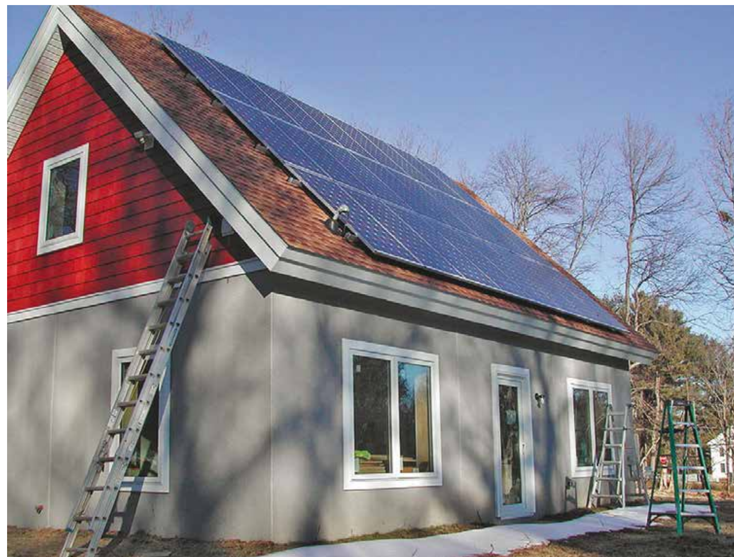
Bargain shopping. Revival Homes’ builder David Jones wanted to change the perception of green homes being only for the affluent by building the Perkins Road House, one that was affordable for the average resident.
