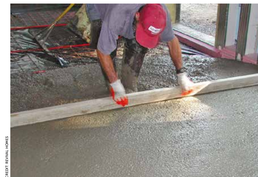
Slab palette. Perkins Road’s concrete slab floor, poured and finished before any interior walls were added, and clear-spanning joists on the second floor allow easy relocation of interior walls in the future.
