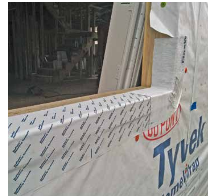
A wall for weather. House wrap is carefully taped and sealed at the edges to provide a continuous weather-resistant barrier under the fiber cement lapped siding.
