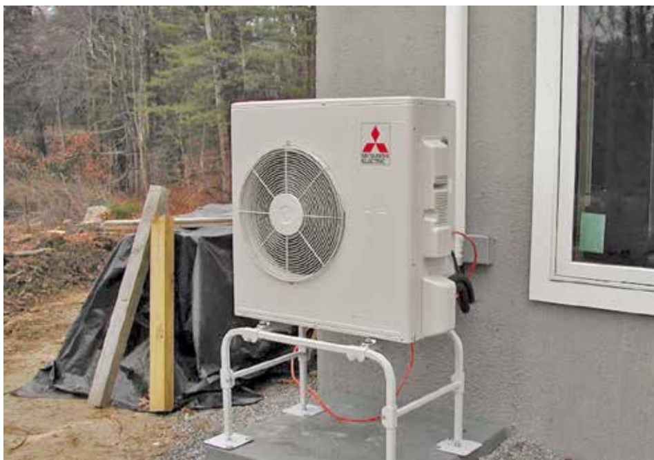
Double duty. A ductless mini-split pump with one inside air handler provides all of the home's heating and cooling.
