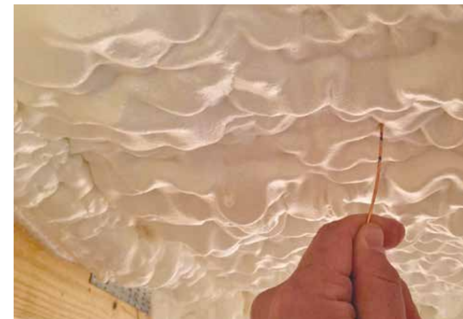
Laying it on. When it comes to insulation, there's no such thing as too thick within the Emery Greenville home.
