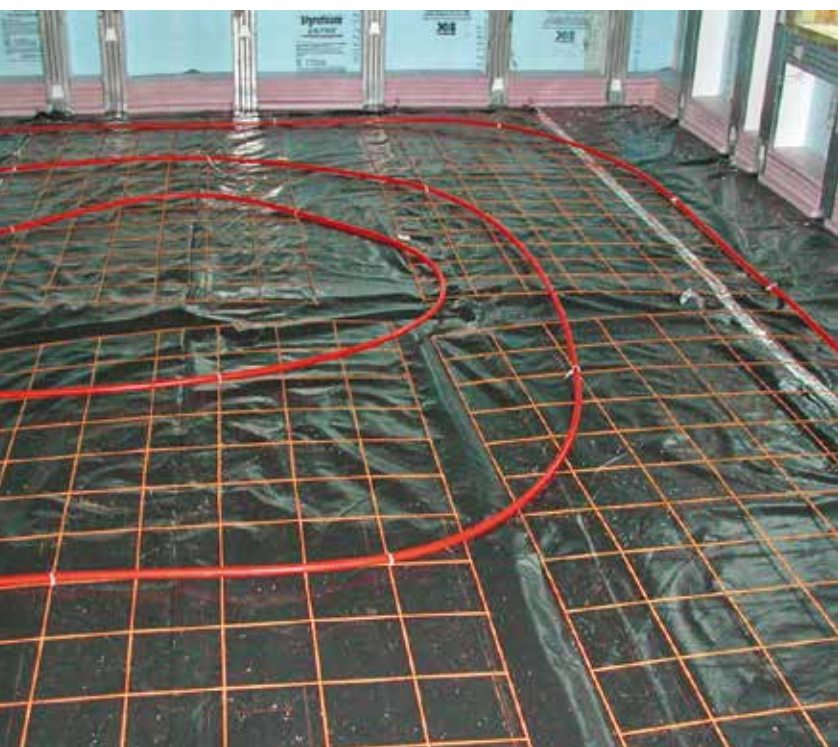
Foot warmers. A polyethylene vapor barrier and loops of PEX tubing are being used to pre-warm well water by as much as 10 to 15 degrees before it reaches the hot water tank.
