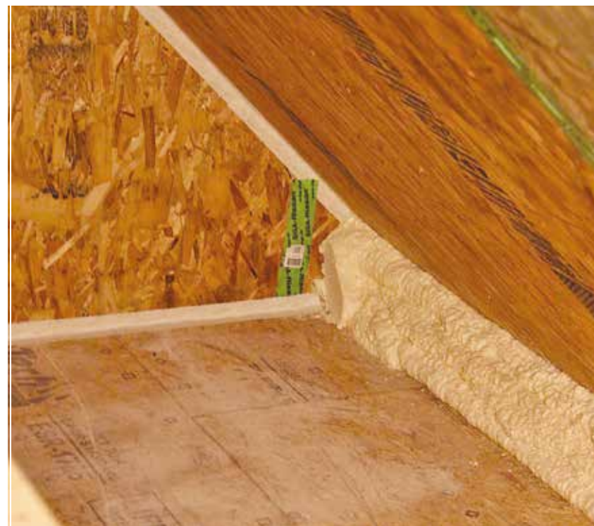
Tight space. The home's narrow roof allows easy install of insulation and sealing agents to prevent moisture and retain temperature-correct air.
