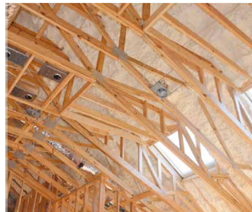
Opening up. The vented attic was ultimately insulated with R-38 blown fiberglass. Skylight shafts were insulated on the attic side with R-10 rigid foam and R-19 unfaced fiberglass batts.
