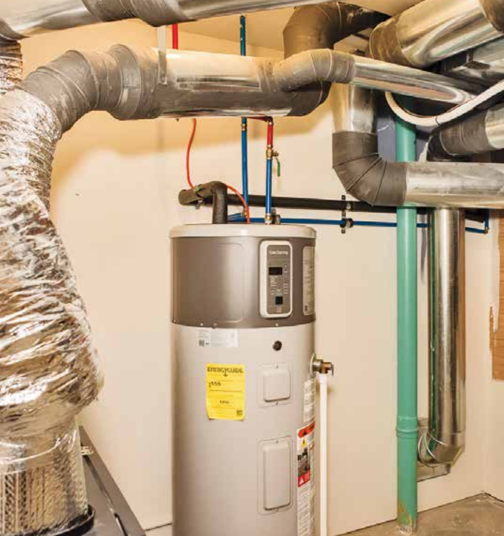
Working parts. A highly efficient GE GeoSpring water heater helps homeowners receive a credit on their monthly utility bill.
