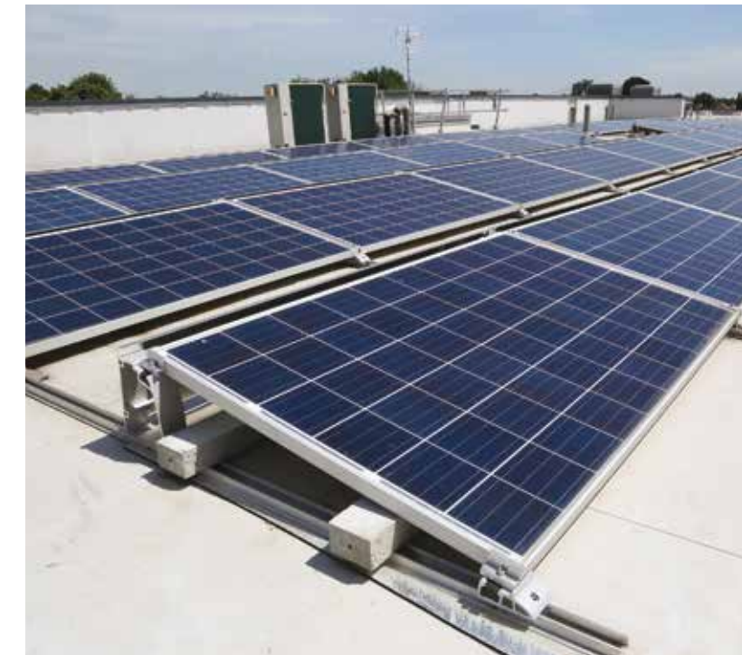
Cooler roofing. Reflective roof membranes over a sandwich of spray foam and Thermax insulation will decouple the mass of the roof from living spaces, while solar panels add another barrier to the sun's relentless heat. This image shows a similar roofing system to the one planned. CREDIT: SIMON TURNER/ALAMY STOCK PHOTO
