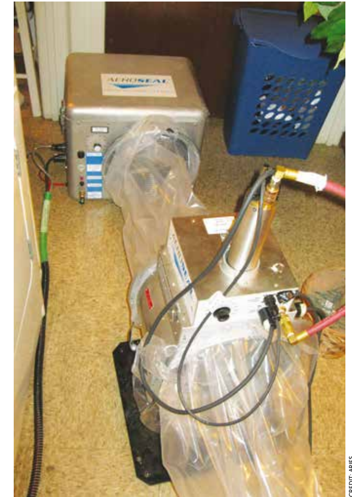
Space Challenged. The plastic tunnel required to inject the Aeroseal sealant into the duct system can be awkward to set up in small spaces.
