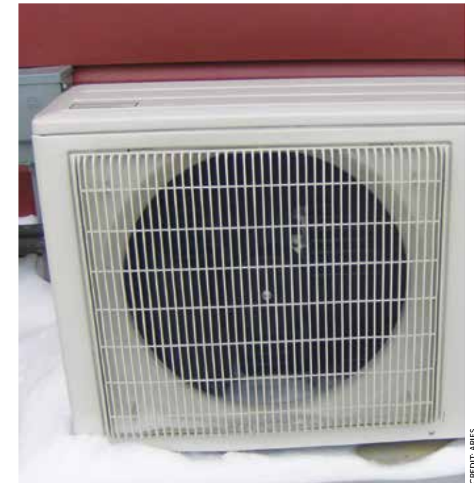
Climate Control. MSHP compressors must be protected from melting snow dripping from roofs above them.
