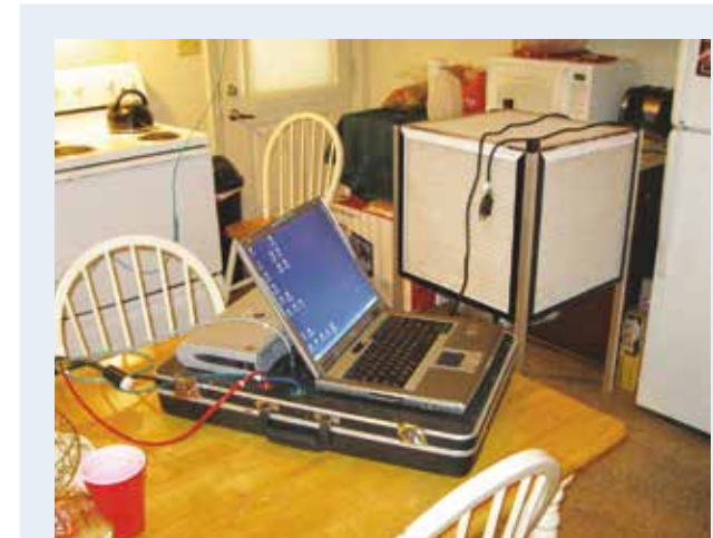
Precise Control. A computer monitors the flow rate, temperature and humidity levels of the air stream, indicating adjustments that need to occur so that the Aeroseal sealant is neither too dry nor too wet when delivered.
