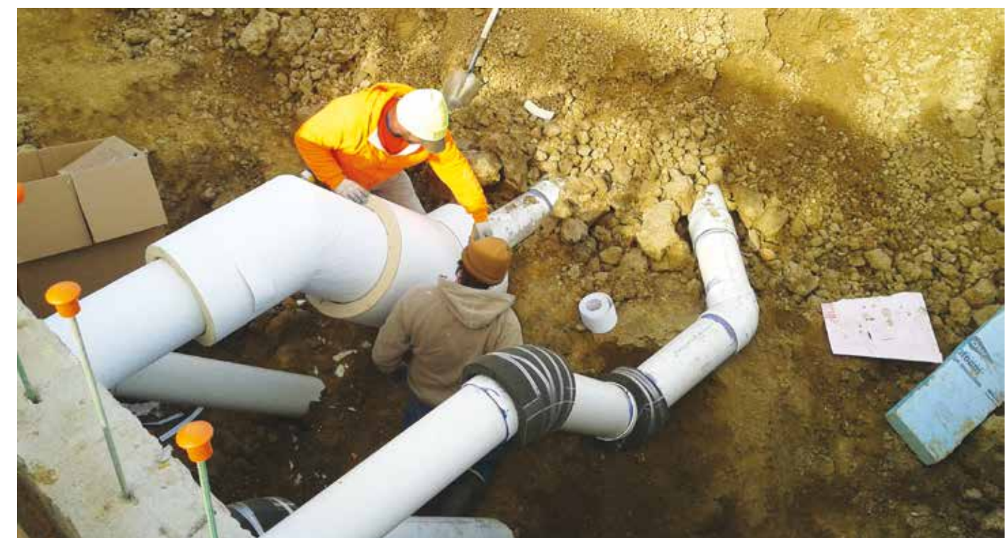
Ground Control. The earth tube system consists of supply and exhaust tubes that connect to energy recovery ventilators (ERVs). The tubes use the constant temperature of the earth to moderate the temperature and humidity of intake air before it passes through the ERVs.
